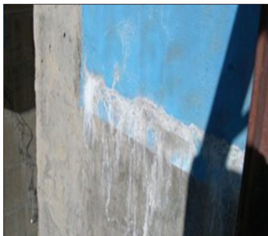
(f) White spots of leaching material on the surface of the walls.
