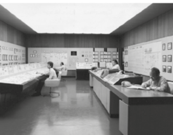
Central Nuclear Juan Domingo Perón (ex Atucha I) Sala de Control
